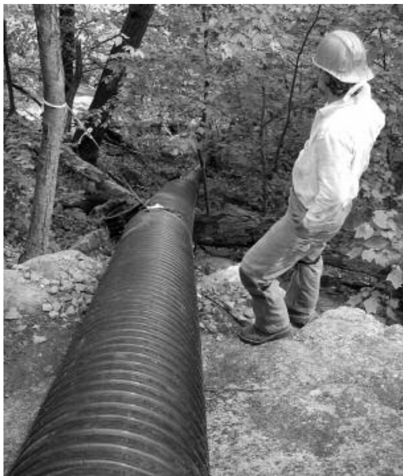
A volunteer monitors the 287-foot long chute used to move material to a work site on Bear Mountain.
